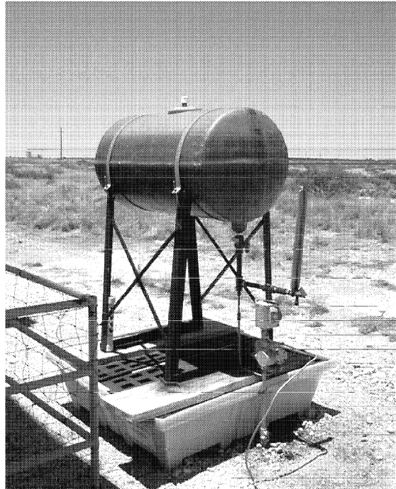
Figure 4. Chemical injection system.
