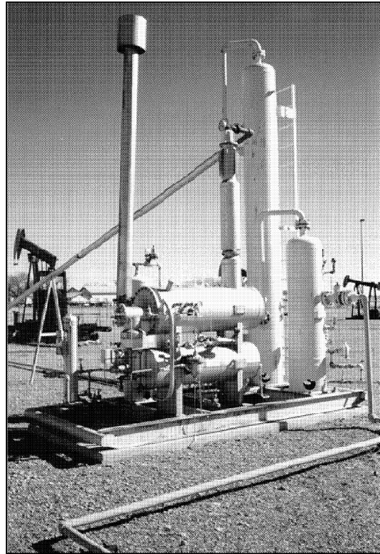
Figure 3. Note the inlet scrubber and contact tower in this view of a dehydration unit.
