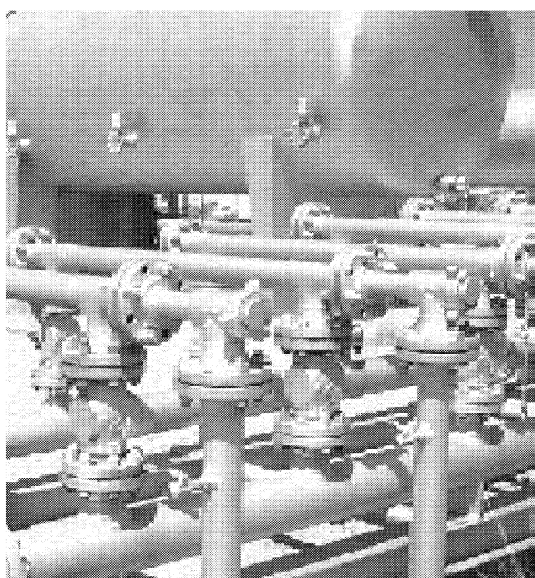
Figure 6. A positive choke installed at the tank battery.
