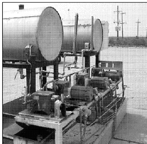
Figure 2. Chemical tanks and injectors set on a concrete base.
