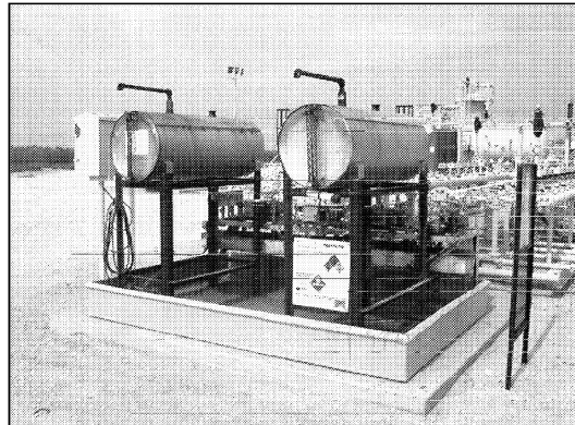
Figure 5. The chemical injection system for a large tank battery with injection at the header.
