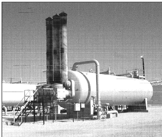
Figure 2. Chem-electric heater/treater for treating crude oil.
