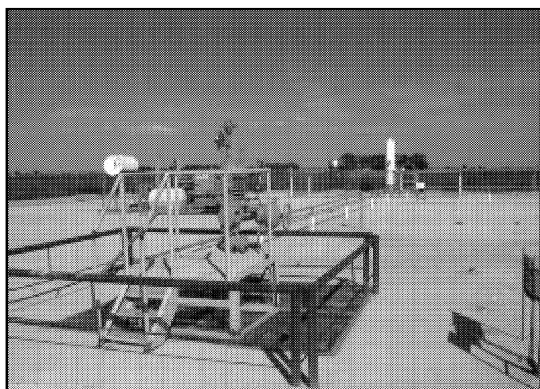
Figure 2. A small gas well with a three-phase separator and compressor in the background.
