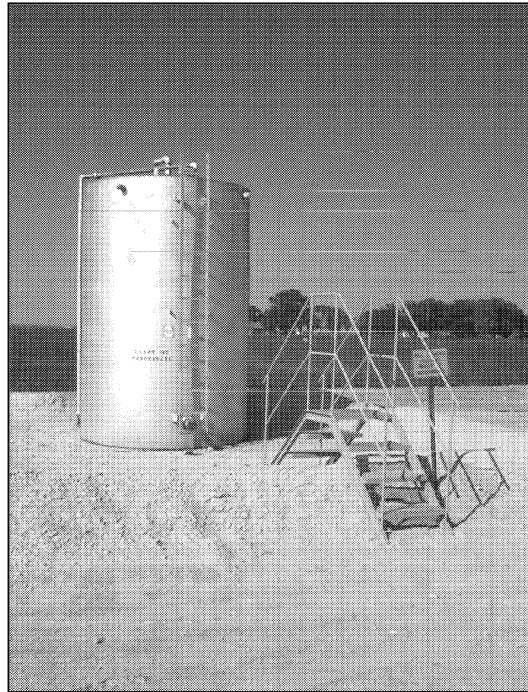
Figure 7. A small tank used to store condensates.
