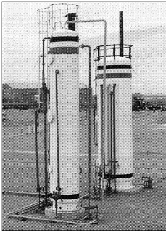
Figure 2. The lines on these heater/treaters are color-coded to identify the fluids they contain.
