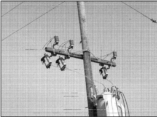
Figure 1. Typical line fuses and step-down transformer common to most leases.
