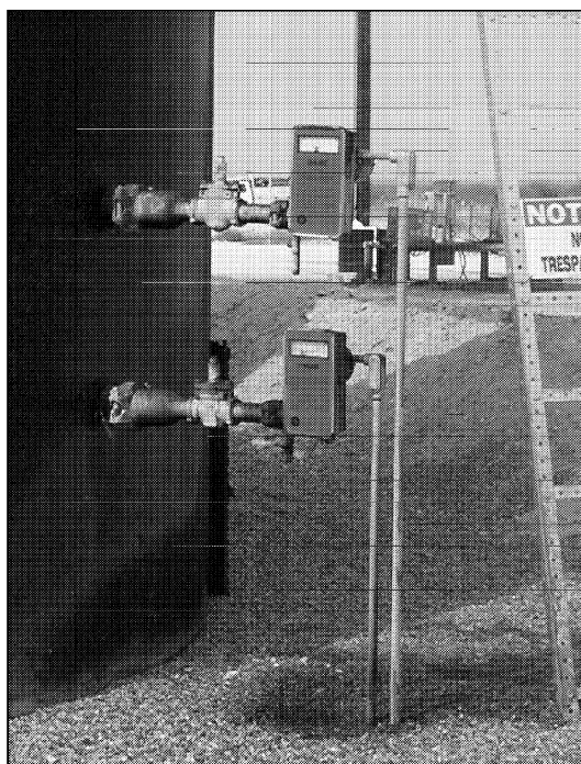
Figure 4. Automatic controls to allow intermittent operation of the water disposal system. Note that a second set of controls is provided as a safety backup.
