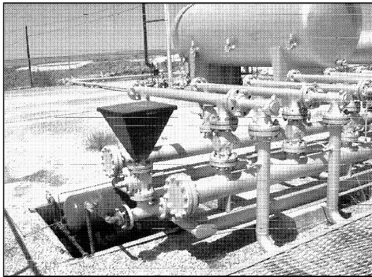
Figure 2. A close up of the header and the oil-saver hopper used on the tank battery shown in Figure 1.
