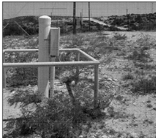
Figure 1. A cathodic protection well.
